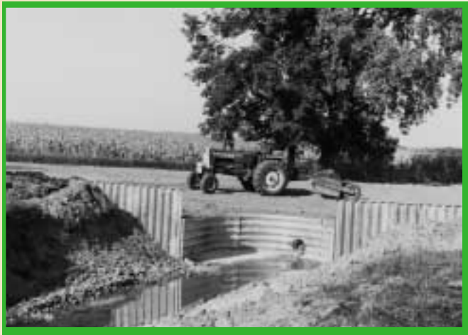
Bill Rawlings doing final grading on a grade stabilization control structure, 1974. Part of Rawlings group project involving seven other landowners.
